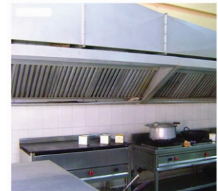
Kitchen Ventilation Systems
